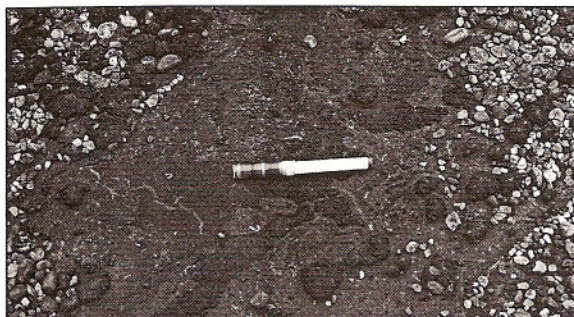
Large blueberry blisters (1.1) and general weather deterioration of (exposed) bitumen (1.10).
